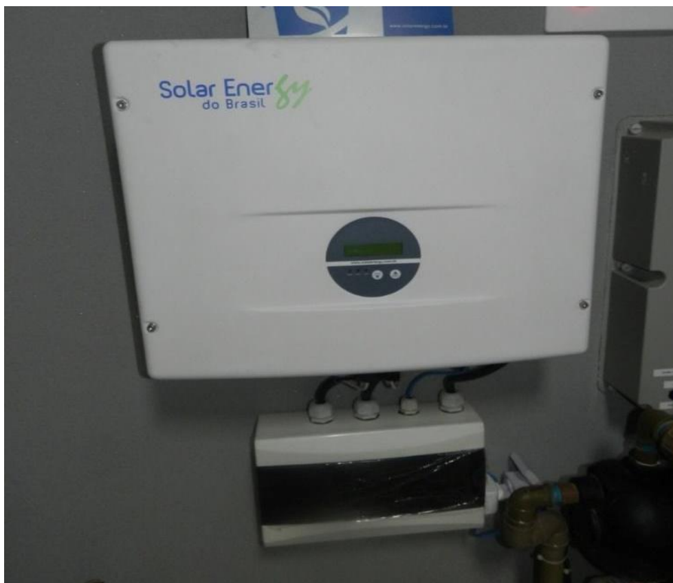
Figura 7 – Inversor de 3 kWp.
